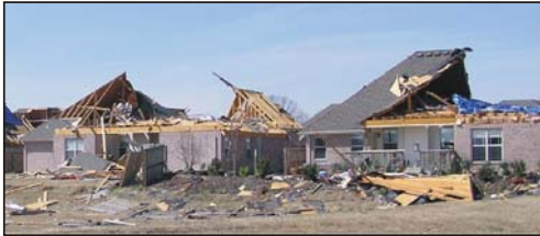
Recent tornado damage at College Place Subdivision.
