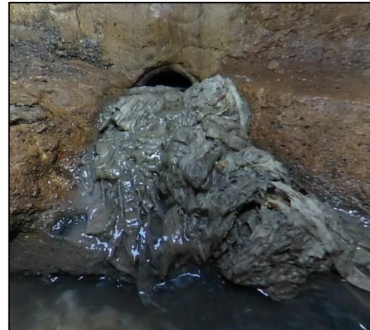
403-586: Debris in Line
